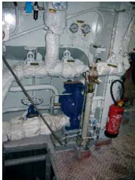
Fuel heater for boiler – Actual location on the ship
